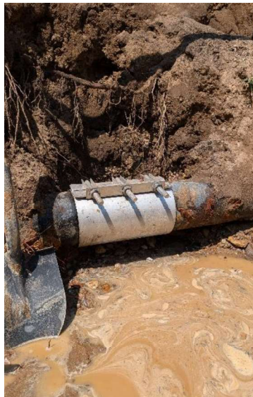
Repair band on the water main at Par Drive
