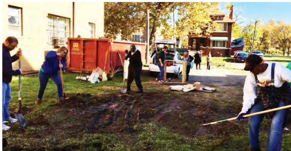
Volunteers worked hard and had fun installing the beautiful vegetation and artwork that make up the rain gardens at the Detroit Library's Duffield Branch.
